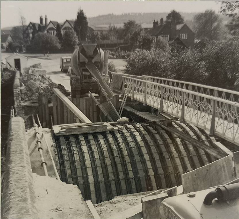
The bridge during channel widening in the early 1960s, with concrete about to be poured.
